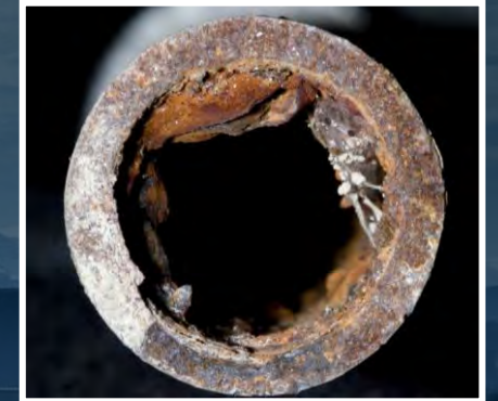
Corroded carbon steel pipeline
